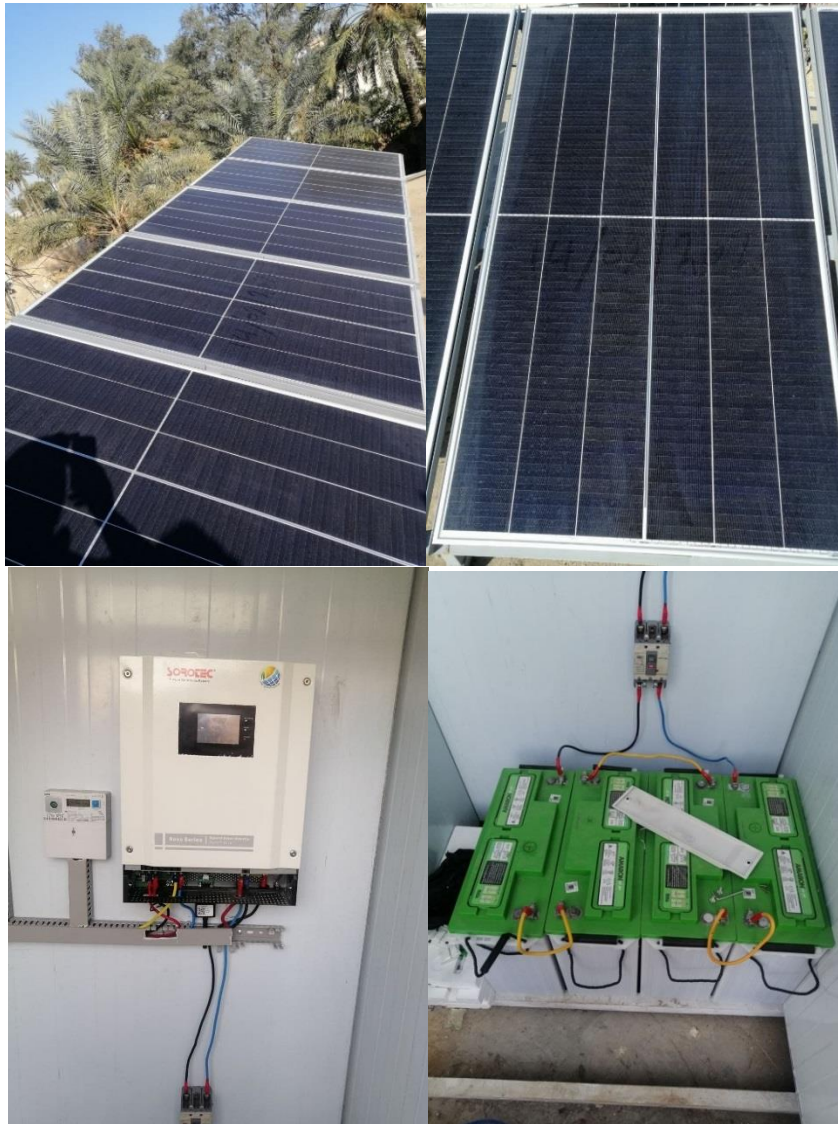
Fig. 1 The installed of PV system
